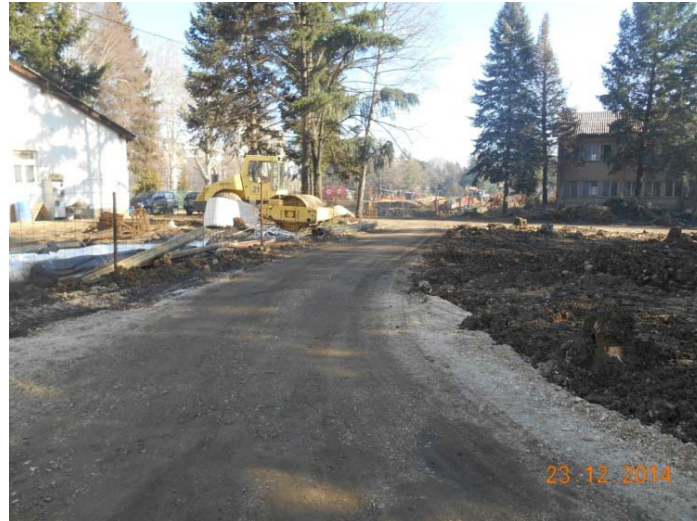
Figure 11 Current condition of the street SrU3 in ARM district 1 Source: CeProSARD's archive
